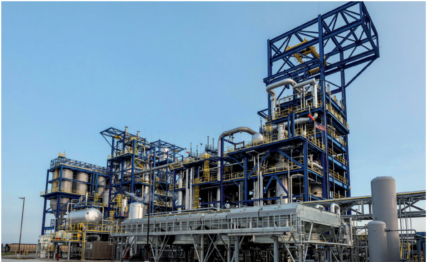
Figure 2 The world's first commercial-scale methane pyrolysis plant
