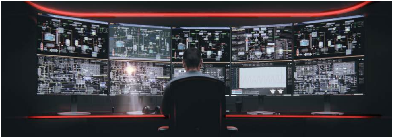
Customer control room
