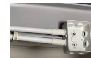
Conduits & electric box from beam
