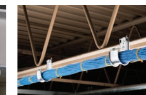
Cables from beam
