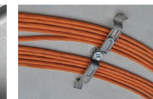
Cables from concrete ceiling/wall
