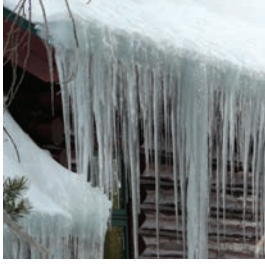
Unprotected roof and gutters
