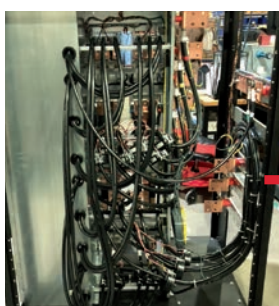
Cabinet with cables
