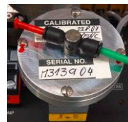
Figure 6 Pressure Test Point
