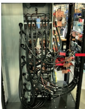
Cabinet with cables
