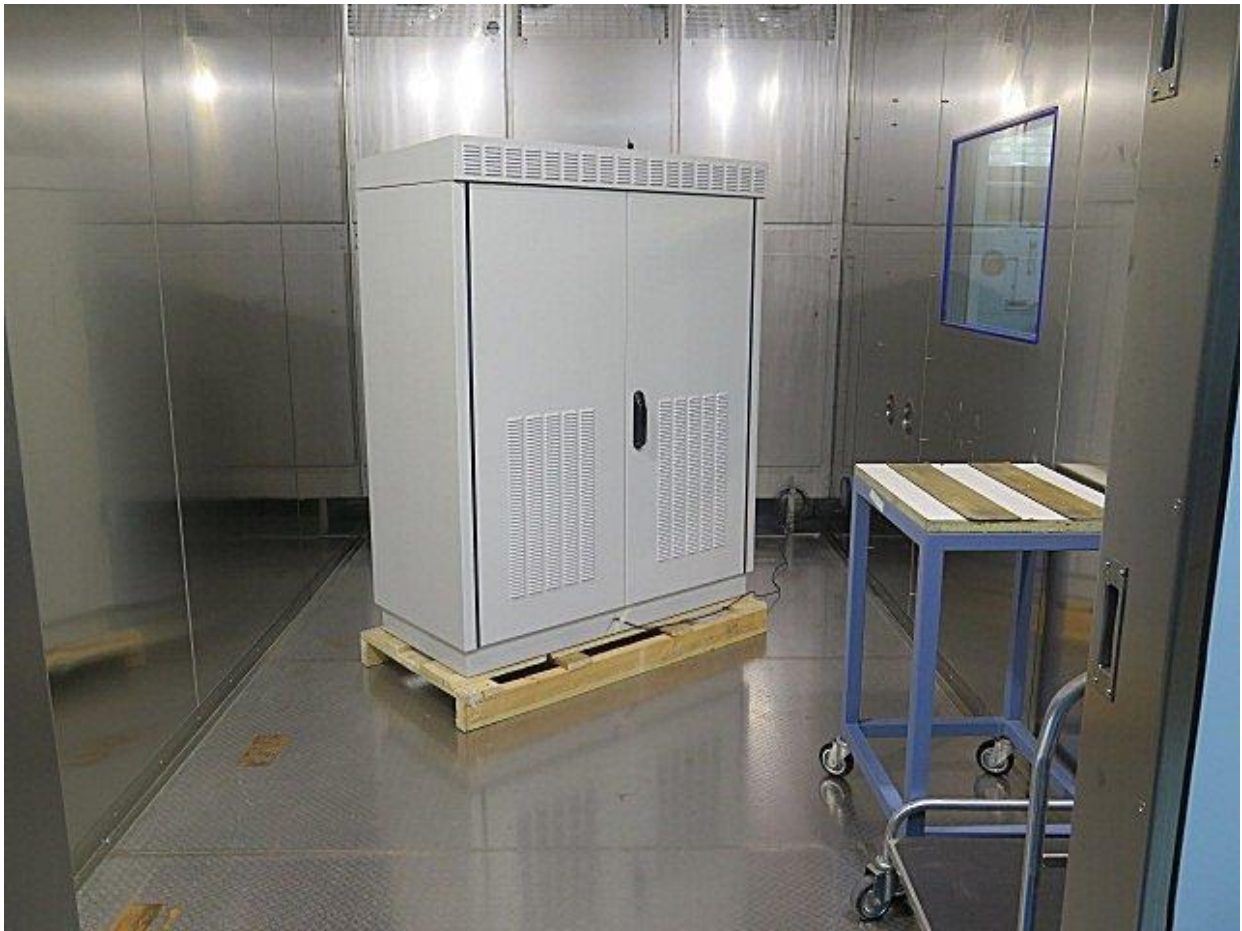
Outdoor cabinet inside the climatic chamber.
