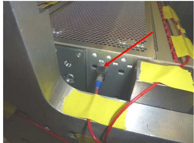
6: measuring point channel 5, right side wall, above
