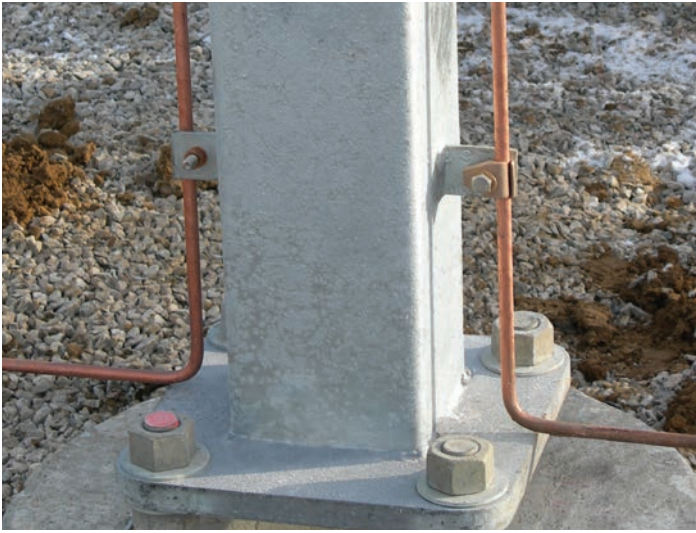
Substation earthing riser
