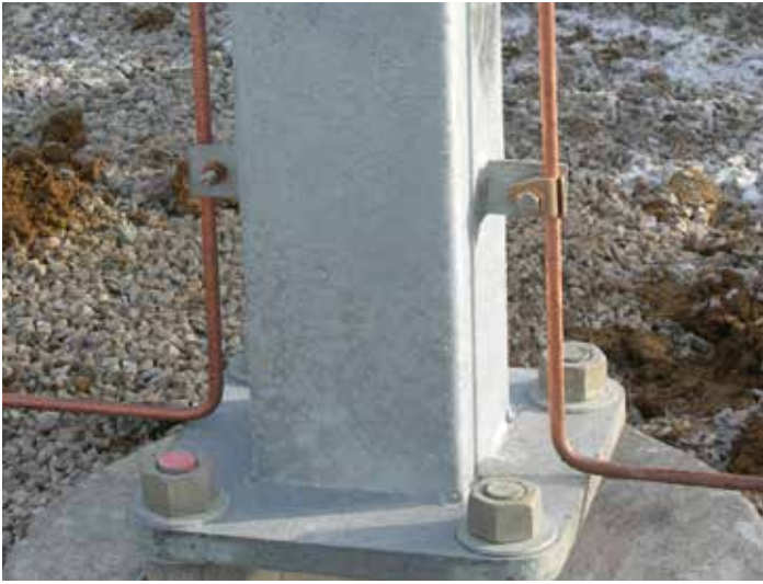
Substation earthing riser
