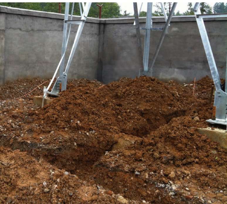
Telecom tower grounding
