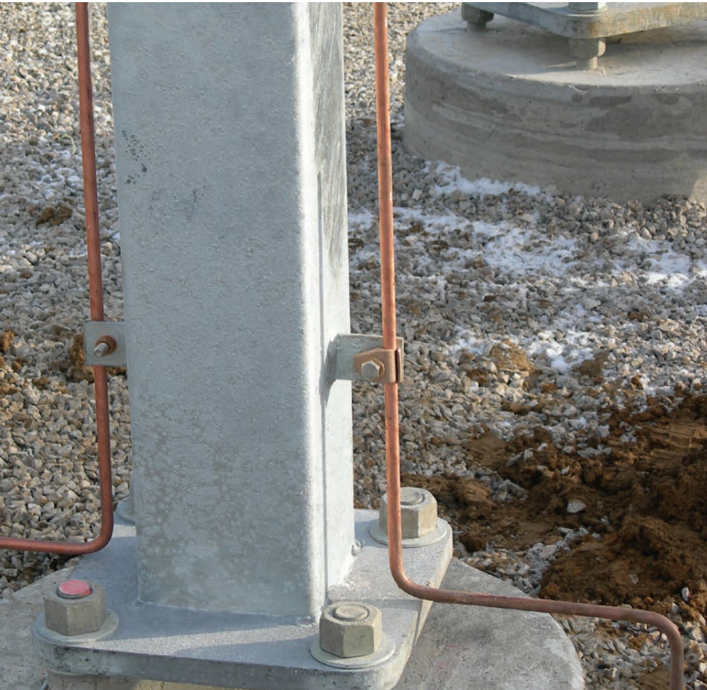
Substation earthing riser
