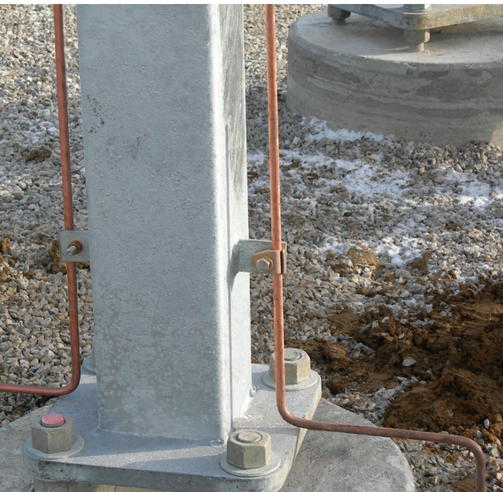
Substation earthing riser
