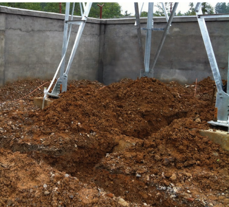
Telecom tower grounding
