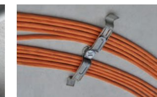
Cables from concrete ceiling / wall
