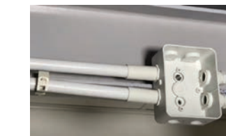
Conduits & electric box from beam
