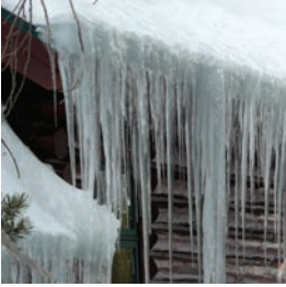
Unprotected roof and gutters
